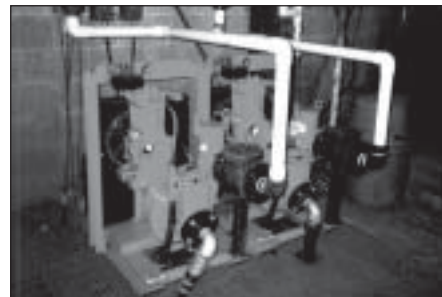
Industrial Wastewater Management – Permanent installation of two 3" (75mm) CD80M electric drive Dri-Prime pumps
